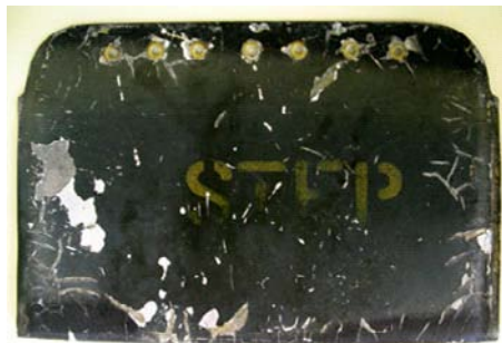
Figure 17. Chinook Fuselage Step Door is shown with flaked, chipped and cracked paint.
